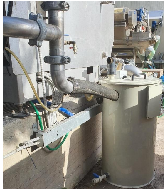
Auxiliary solids recovery tank
